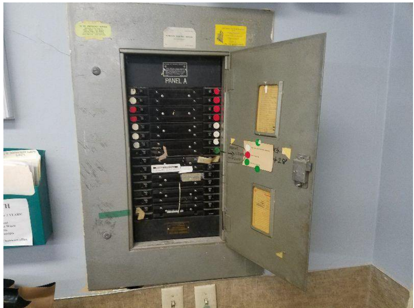
This panel a is downstairs in the main room near the janitor closet.
