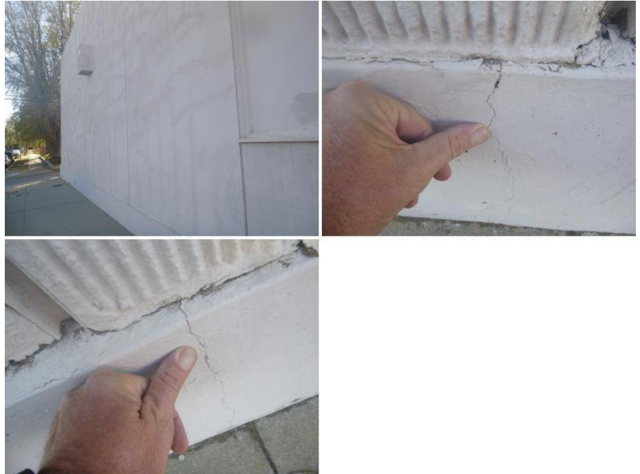
There are many small hairline cracks along the foundation footing visible along the left sidewalk area. These do not appear significant..
