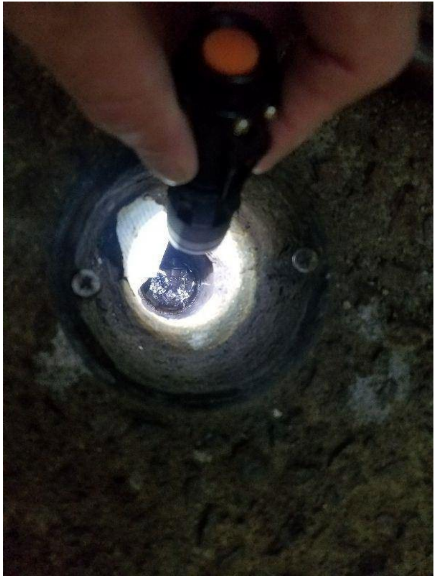
Needs Attention: Older drain lines under slab, seem at floor drain in janitor closet.
