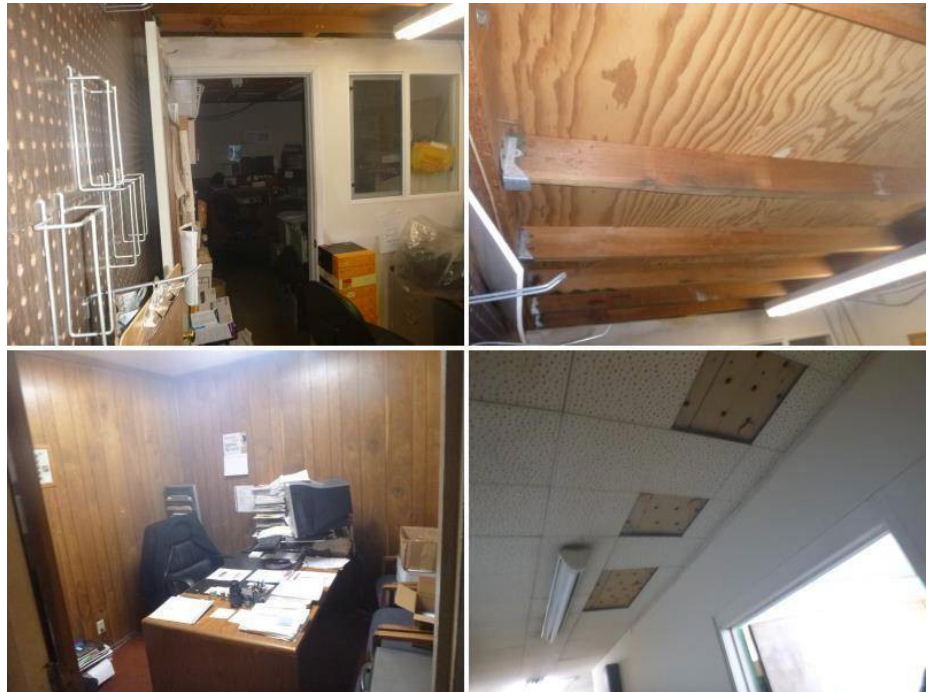
Note light duty 2x4 supports are used for the mezzanine floor supports.
