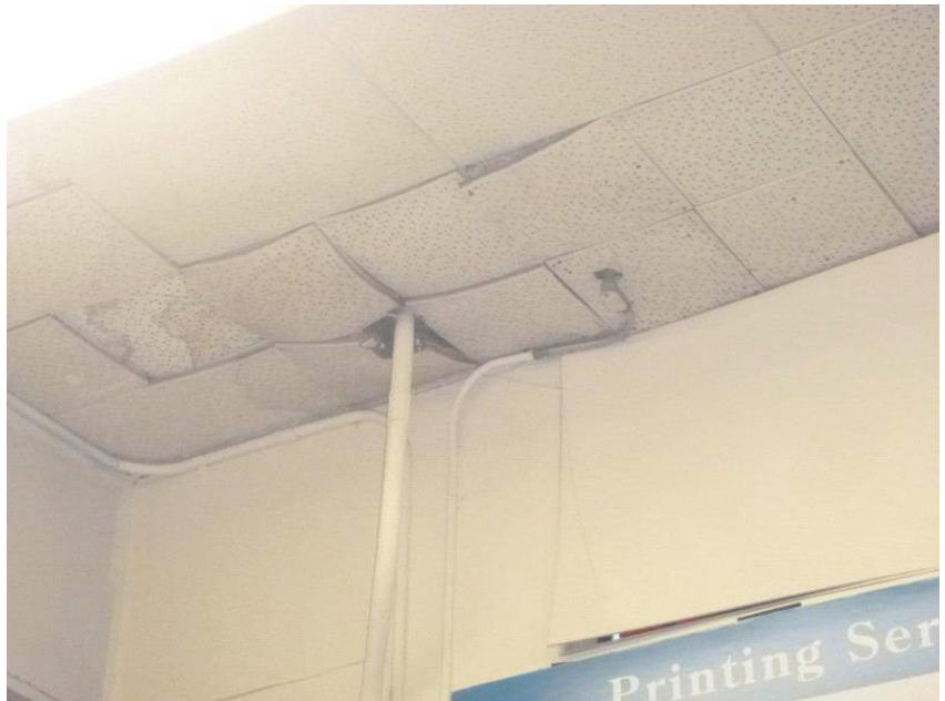
Needs Attention: CEILING: There are areas of moisture stains on the ceiling near the front left corner where the roof drain comes down through the building.
