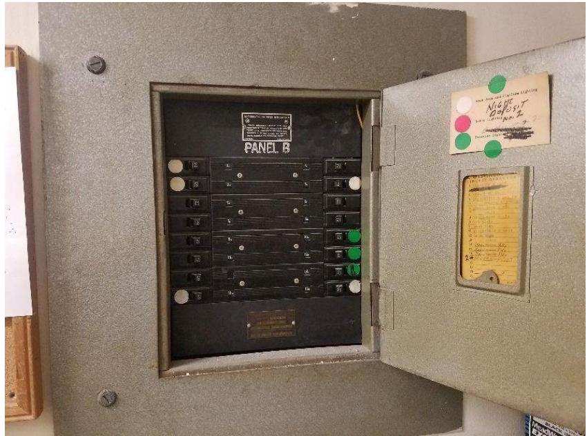
This sub panel B is upstairs in the hallway.
