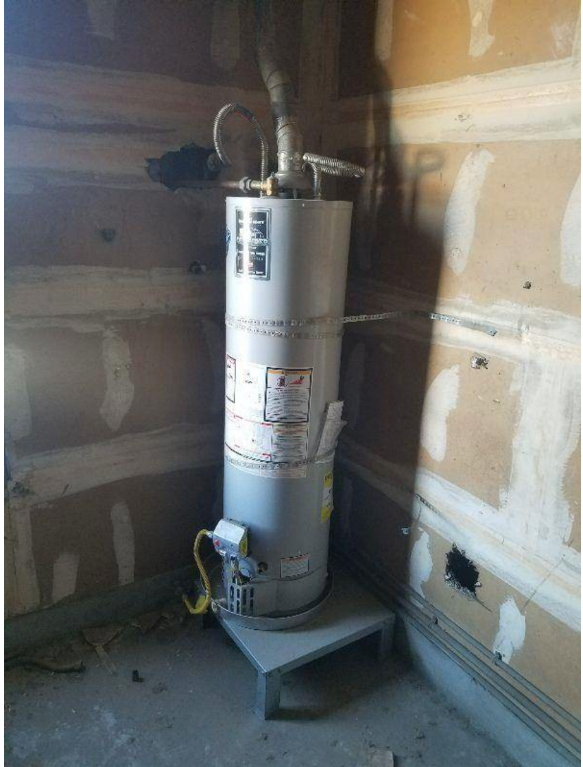
The water heater is located in the roof closet.
