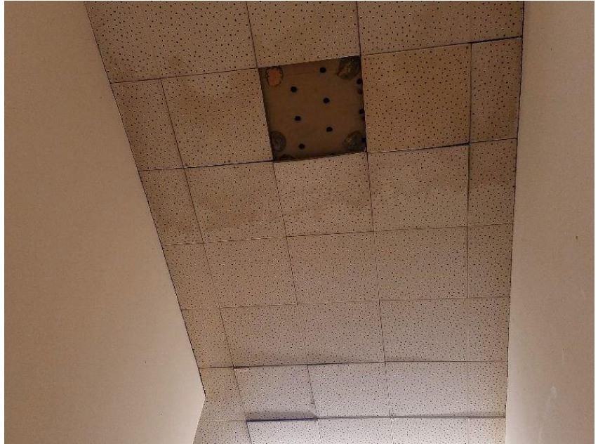
CEILING: There are areas of moisture stains on the ceiling above the stairs.(below the old roof utility room)
